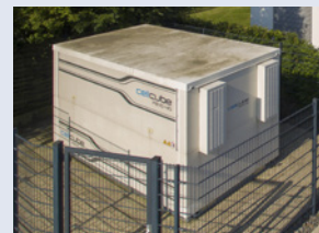
Central electricity storage
