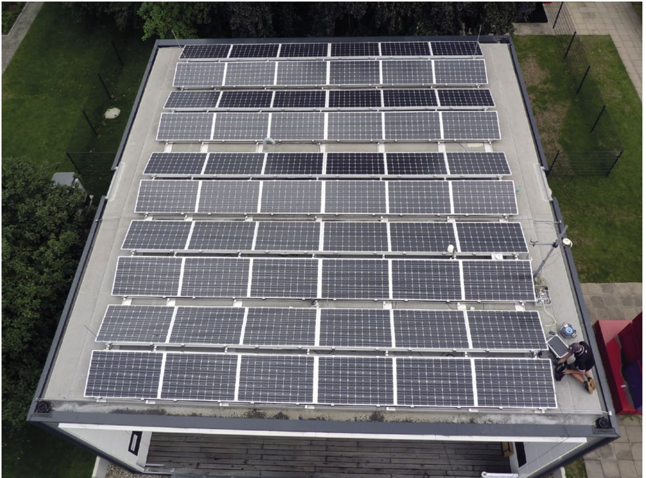
Roof area with monocrystalline photovoltaic modules
