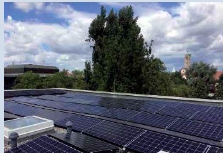
Figure 12: The photovoltaic system Photograph: Rhine-Neckar District
