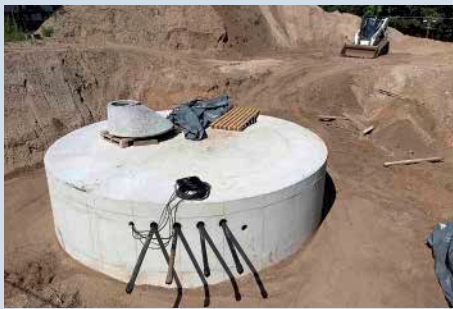
Figure 11: The ice storage unit during construction Photograph: Ingenieurbüro Willhaug Gebäude- technik GmbH
