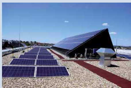
Figure 23: PV system on the roof of the new build Photograph: Neutraubling Upper Secondary School
