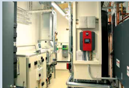
Figure 71: The plant room Photograph: Haase & Bey Architekten
