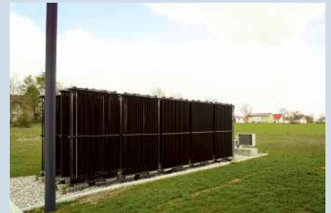
Figure 60: The solar air absorber block Photograph: City of Feuchtwangen
