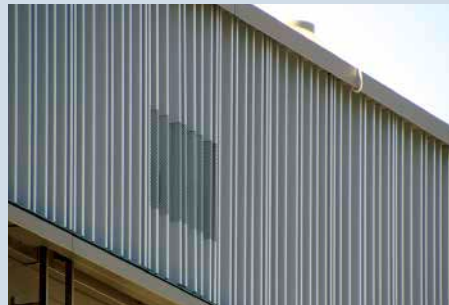
Figure 47: Detailed view of the façade showing the air inlets/outlets Photograph: Town of Kaufbeuren
