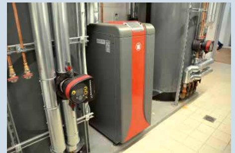
Figure 72: Heat pump and stratified storage tank Photograph: Haase & Bey Architekten
