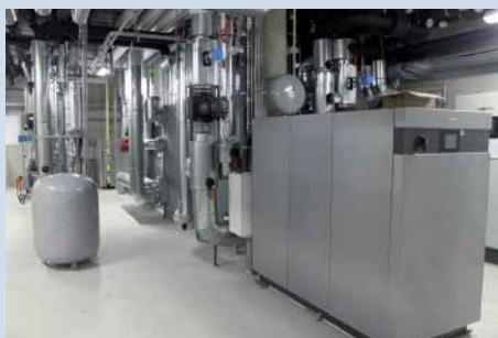
Figure 35: The heat pump in the plant room Photograph: COPLAN AG
