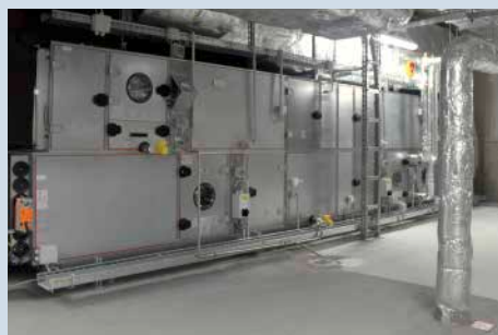
Figure 34: The central ventilation system Photograph: COPLAN AG
