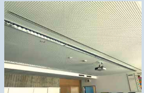
Figure 48: Supply air slot diffusers in the ceilings Photograph: Güttinger Ingenieure
