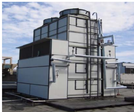
Figure 6.1: Principle of the indirect evaporative chiller (left) and picture of the first developed unit (right).
